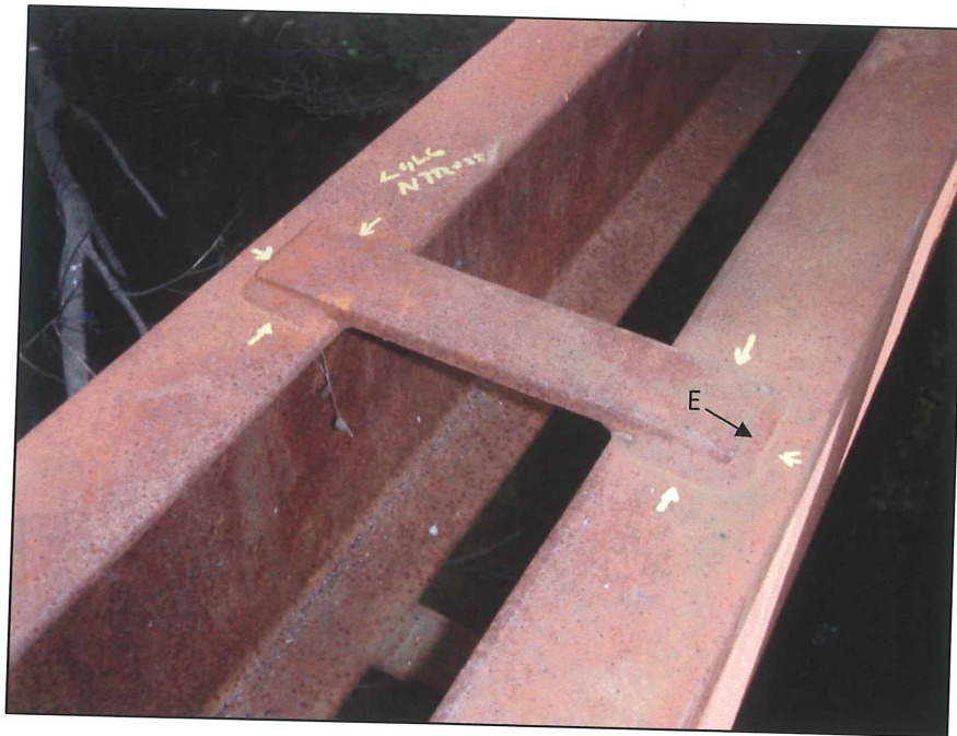
Figure 7 – Looking at L4-L6, north truss. Note: Welded attachments on the top and bottom flanges of the lower chord.
